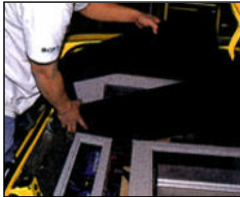
29 – At this point, everything was installed and the only thing left to do was fabricate and upholster various trim panels like this one that filled in the passenger's side of the trunk and framed the changer.
