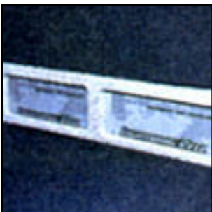
27 – A trim panel, covered in more of that black carpet, finishes off the batteries.
