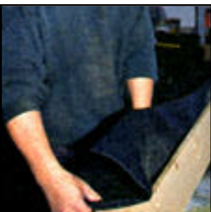
17 – Once the carpet had been laid into the tray and smoothed up onto the walls, a sharp razor knife makes easy work of trimming the excess material.
