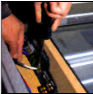
12 – One by one each of the terminals on the amps was filled with the appropriate wire.
