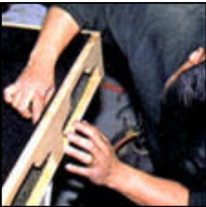
5 - A sharp razor blade makes trimming the non-backed carpet a snap—although safety should always be an installer's first concern. This part of the amp rack sits toward the front of the vehicle and as you can see by the shape, the Tube Driver amps will actually protrude through this part of the rack.
