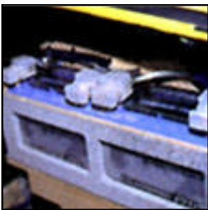
26 – Next, the box was covered with a layer of tweed and the batteries were wired with no less than Lightning Audio's finest 4-gauge and accessories.
