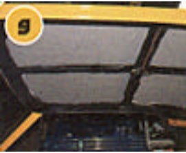
9 – When working overhead like this it is a good idea to cover the floor and anything else you don't want mud to fall on.
